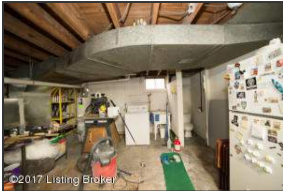
The unfinished basement provides for a desirable space for additional storage, hook ups for washer/dryer, utility sink and toilet
