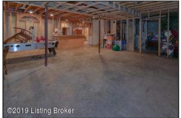
The basement has recently been framed with electric and plumbing installed (the shower has already been installed too) and is ready to be finished with flooring and drywall to complete the final touches!
