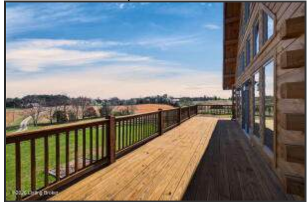
The expansive back deck runs the full width of the home and looks out over open Kentucky land
