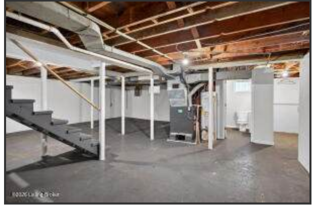
The HVAC and water heater are housed in the basement
