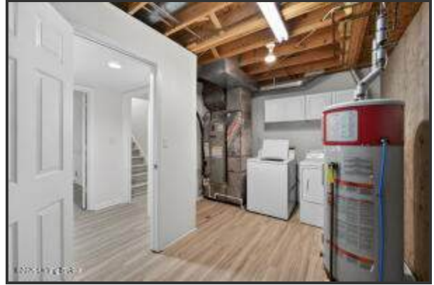
Lower Level: Utility Room
